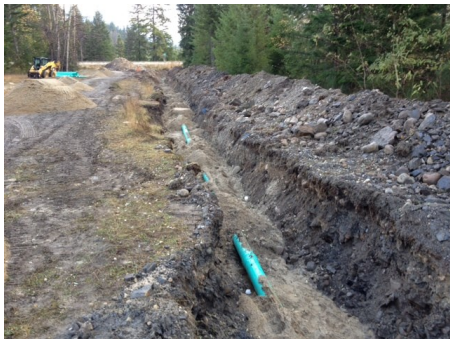
Projects (left to right): .Sewer line relocation, Nakusp Airport improvements, completion of the Water Treatment Plant
