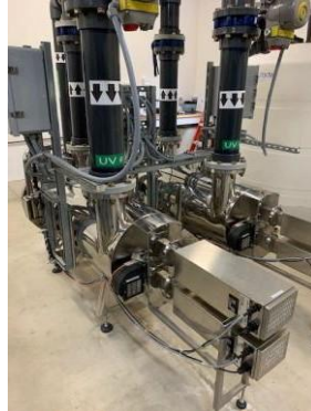
WTP UV System
