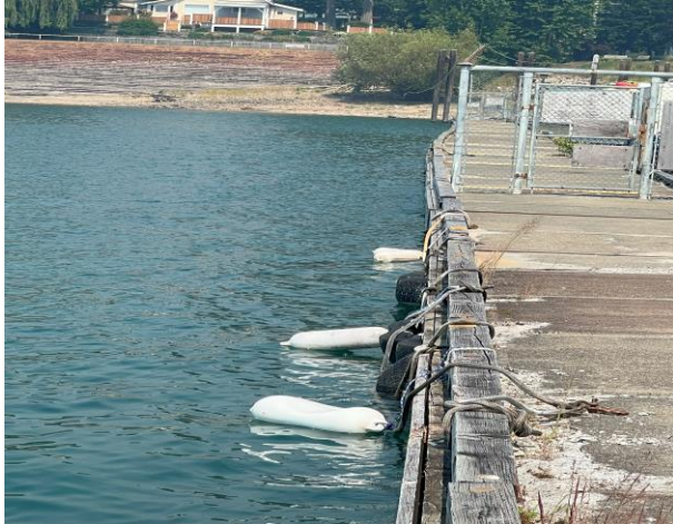
Bend in floating dock walkway
