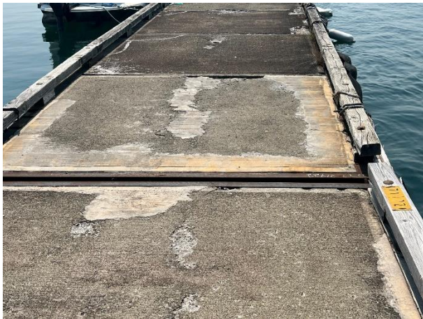
Slip 71 unattached and broken concrete
