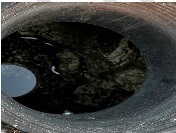
Access hole filled with water
