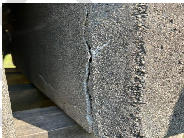
Concrete cracking between fourth piling
