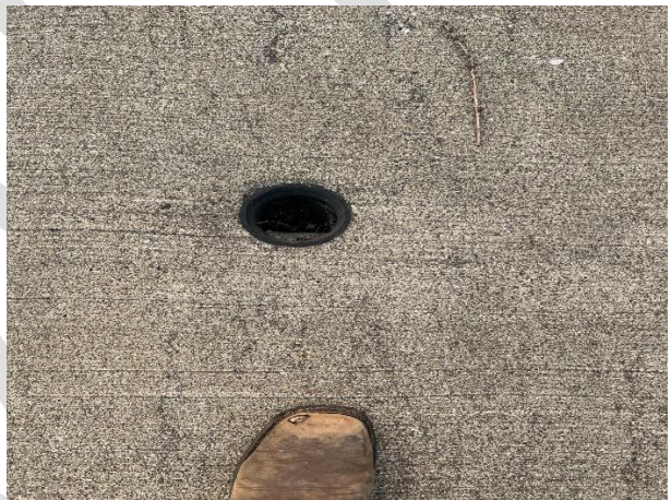
Missing access hole plugs
