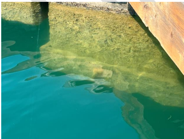
Exposed foam floats on south sections
