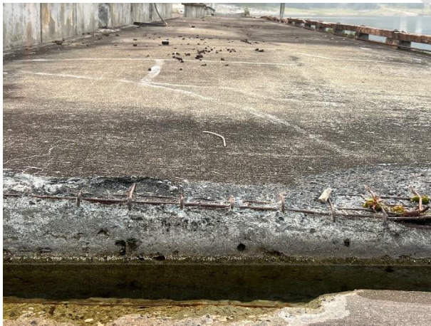
South breakwater heaving
