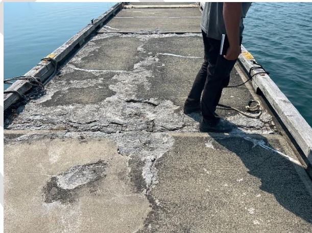
Concrete walkway showing damage
